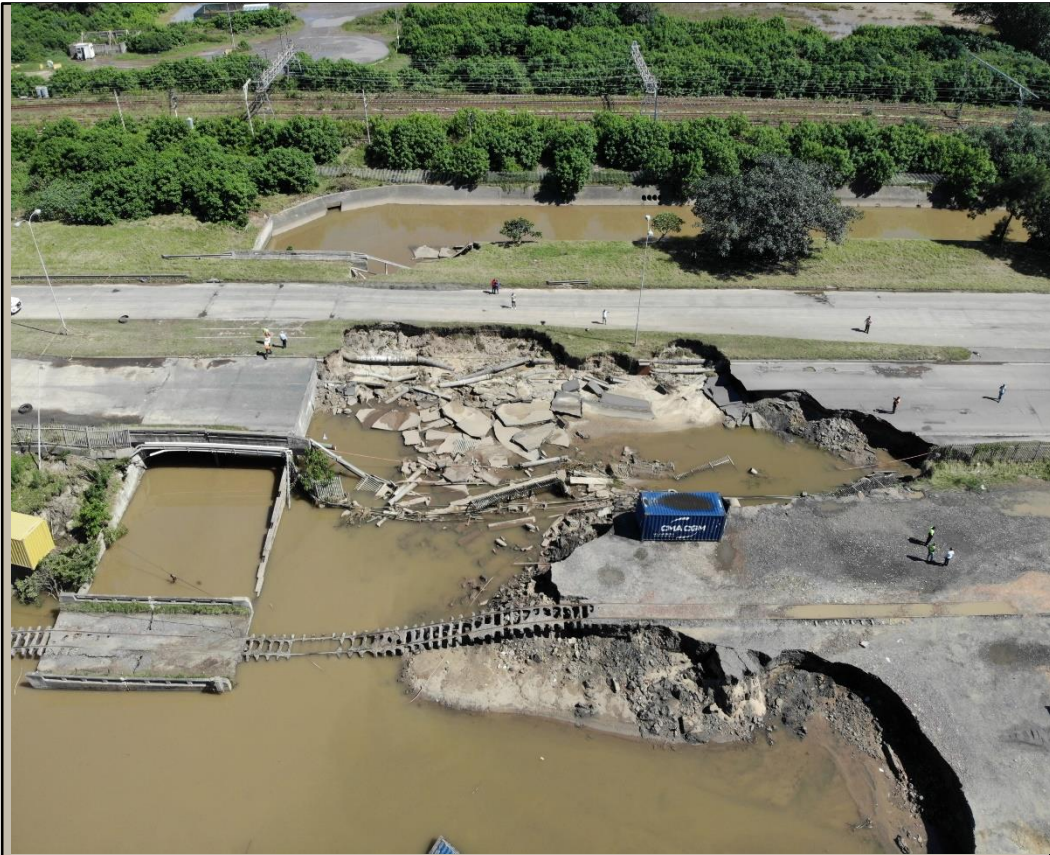
Damaged section of Bayhead Road: 14 April 2022
