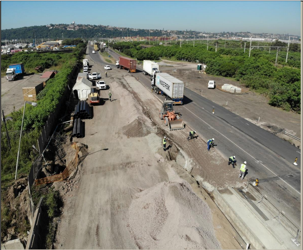
Damaged section of Bayhead Road: 06 May 2022
